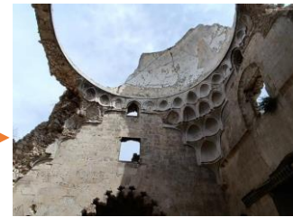
Figure 10. Increased deterioration in the dome of the great hall
