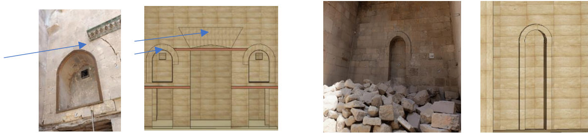
Small stone arches hold the pressure from the stones above the stone windows and doors
