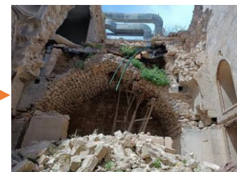
Figure 16. Complete collapse of the western wall of the large hall
