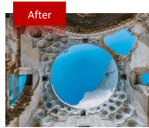
Figure 9. A major collapse in the dome of the large hall
