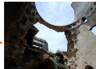
Figure 13. Collapse of the Northwest corner apse
