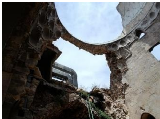
Figure 13. Collapse of the northwest corner apse.
