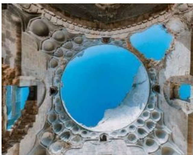
Figure 9. Major collapse in the dome of the large hall after the war.
