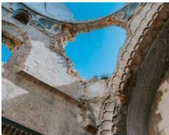
Figure 12. Collapse of the southeast corner apse.
