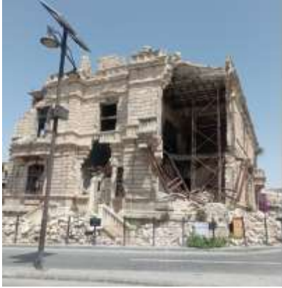
Figure 2: west and partial collapse in south west façade- Department of Immigration
